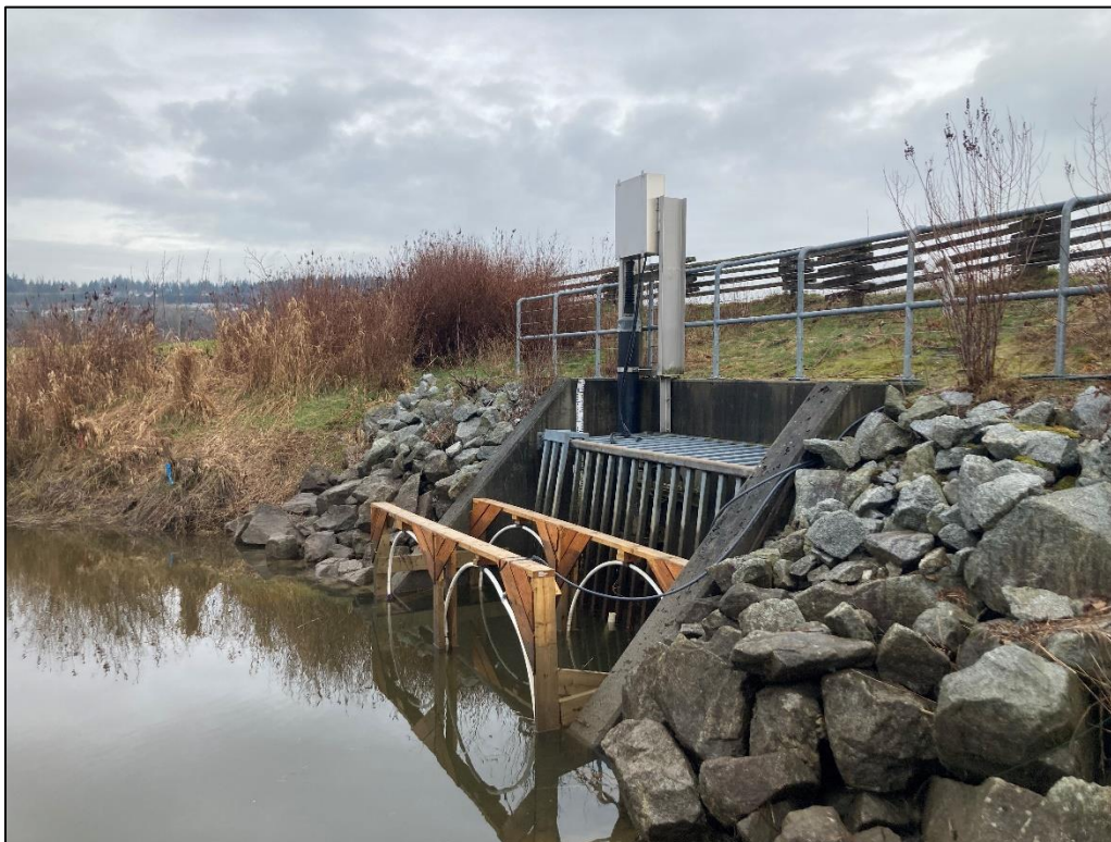
Figure 6: Antenna installation with lumber frame in final position at self-regulating gate. Photo by: Zachary Sherker, project lead
