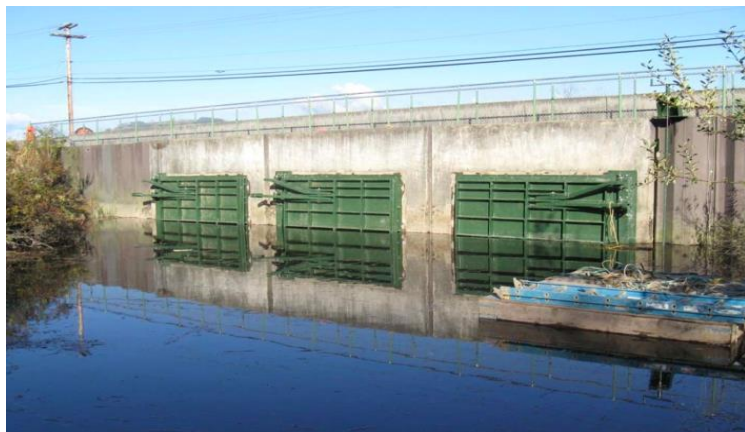
Side-hinged tide/floodgate array by Nehalem Marine Manufacturing 10
