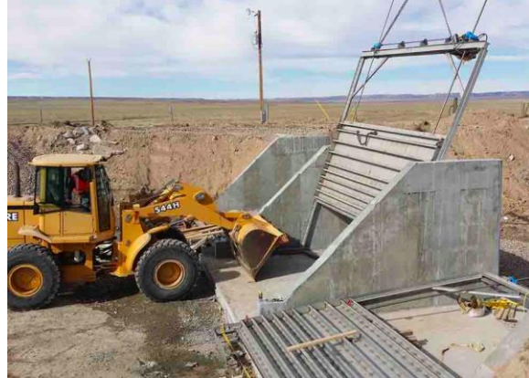
Vertical sluice gate installation by Watch Technologie 9
